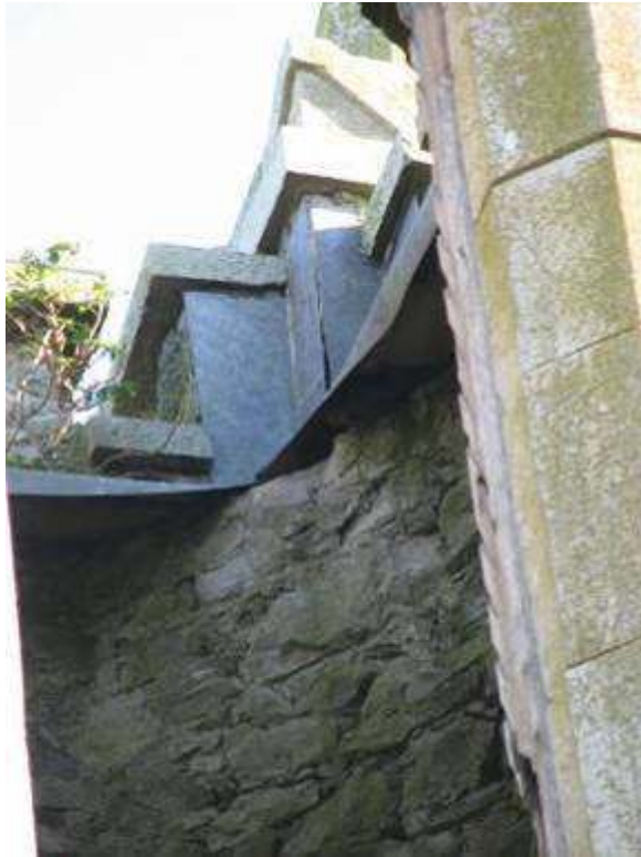
Detail behind parapet (note unsupported lead gutter lining)
