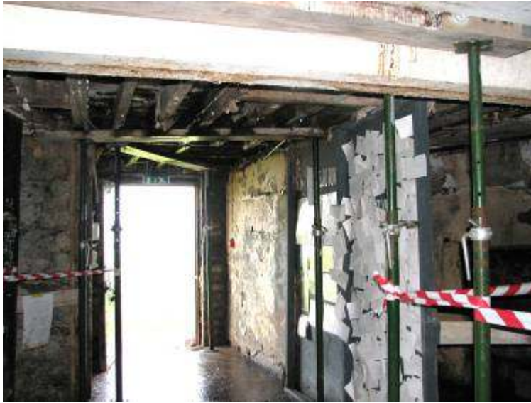
Interior – ground floor – note propping of floor over
