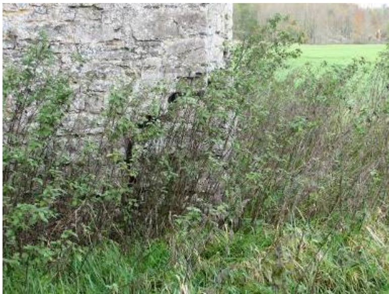
Subsidence at South-East corner
