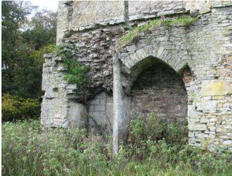
East wall – damaged arch springing and missing voussoirs
