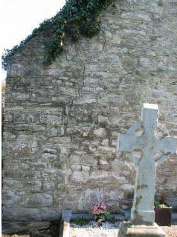
Cracking on east gable (note graves directly beside the wall)
