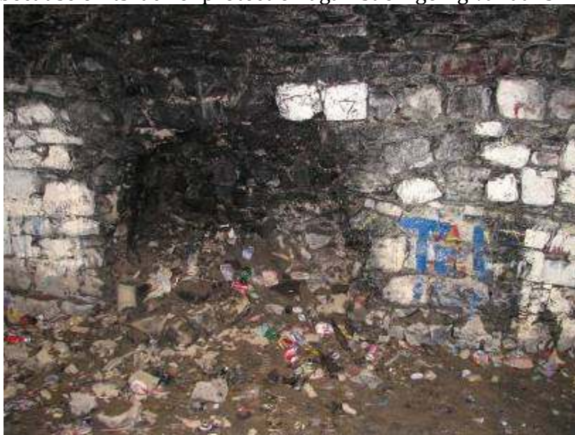
Undercroft – collapsed fireplace
