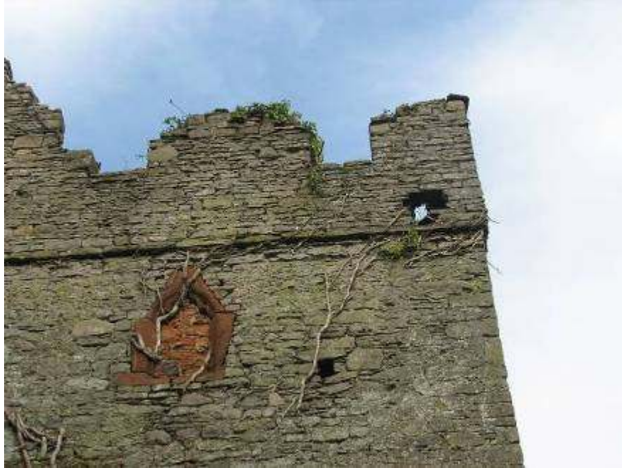
Hole in masonry at south-east corner
