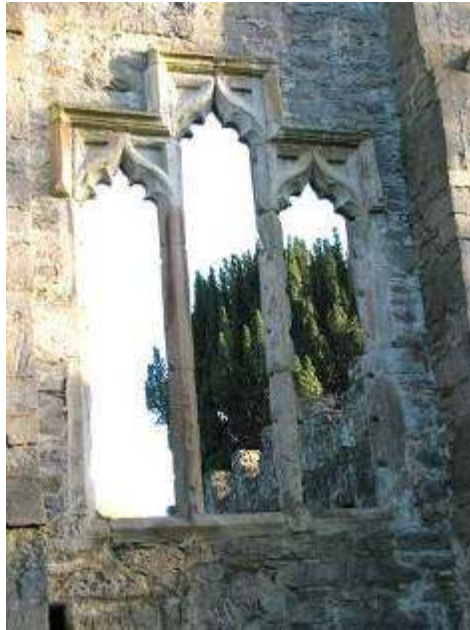
Detail of west window – note damage to mullions
