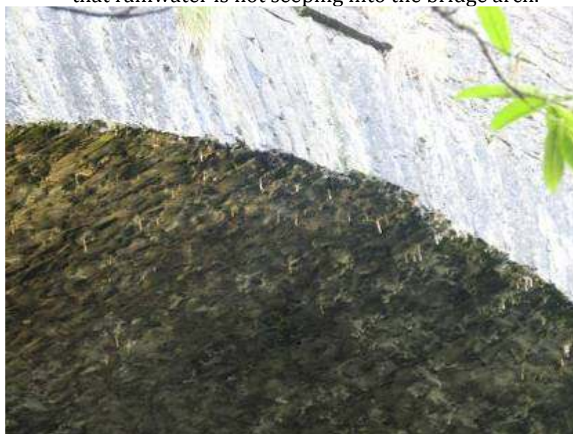
Lime 'stalactites' on bridge soffit
