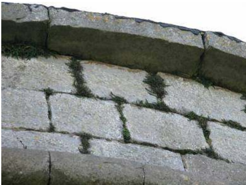
Evidence of water ingress at high level
