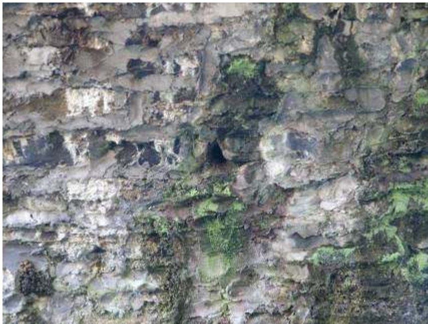
Possible hole in bridge soffit
