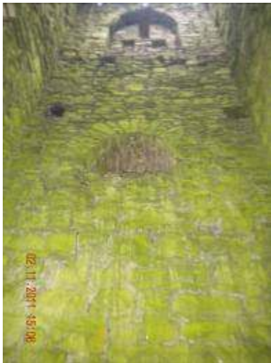
Green mould on the interior of the tower wall
