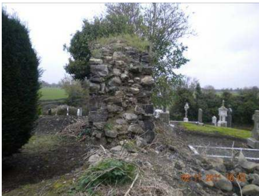
North end of West wall (note the wall leans to the West)
