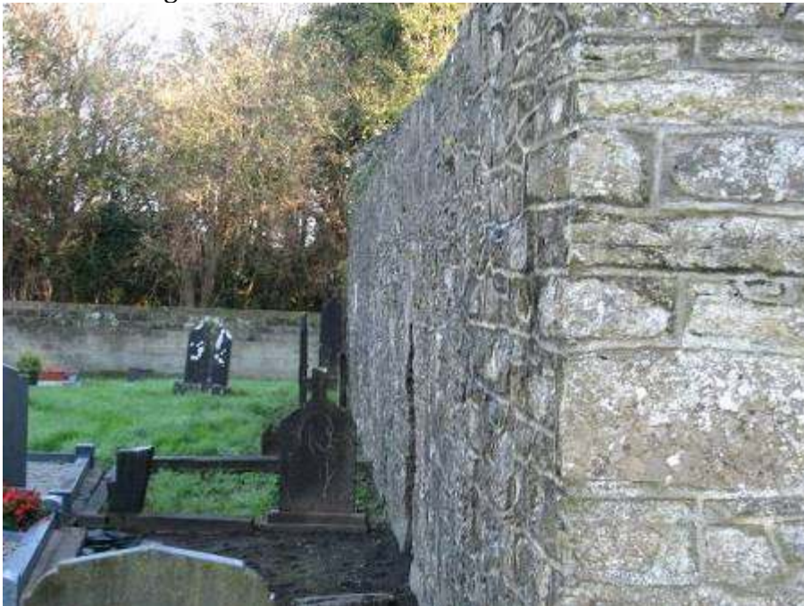
View along north wall (note bulging)
