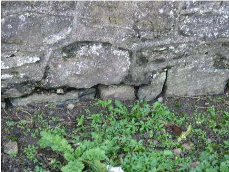
Mortar washout at the base of the north wall
