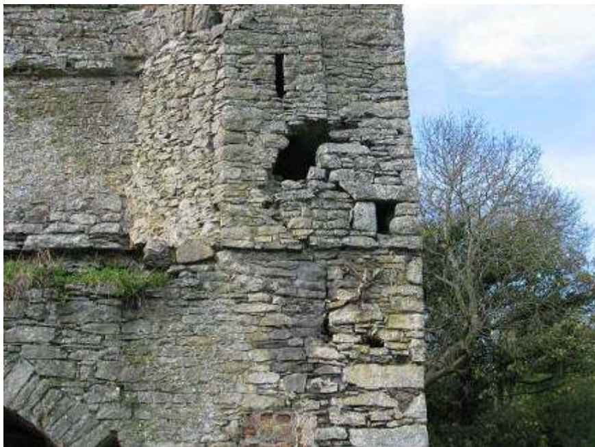
North-East corner bulge and hole – east side
