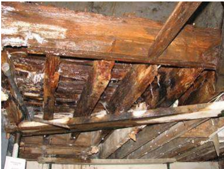
Ground floor – note rotted timber floor over
