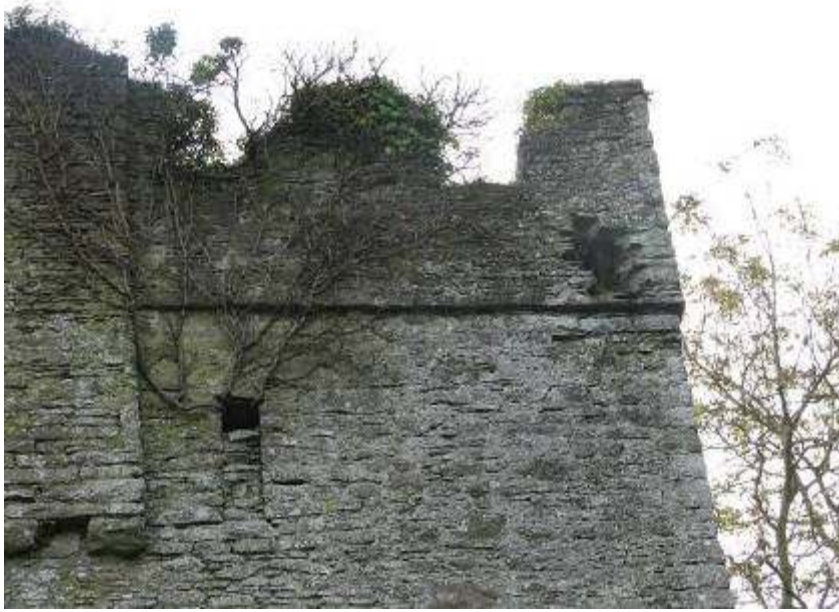
Hole in masonry at north-west corner
