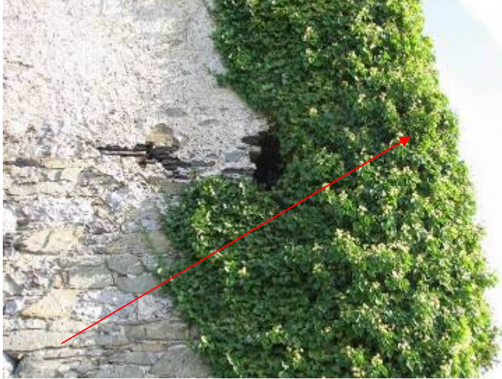
Hole in south-west corner partly hidden by ivy
