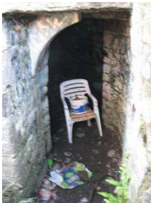
Entrance to undercroft (note damaged arch)
