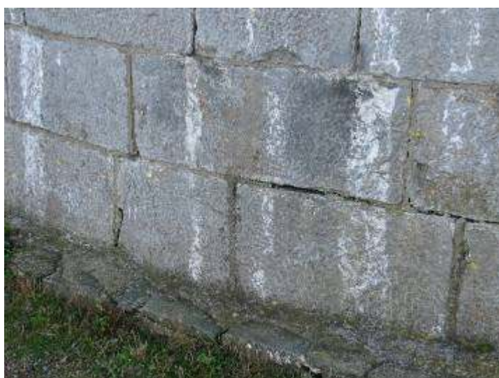
Evidence of mortar washout at low level
