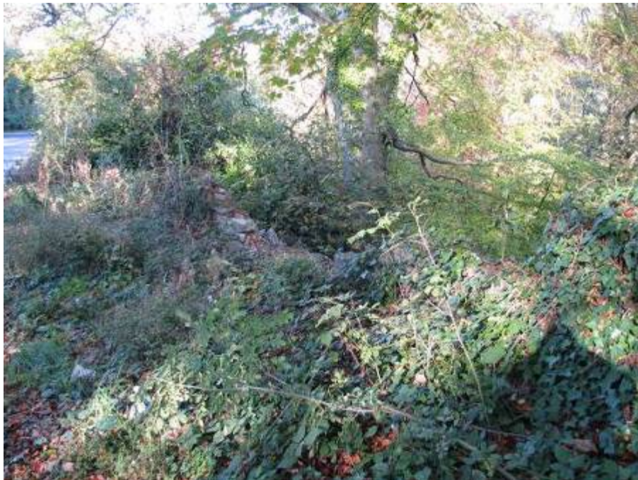
Collision damaged wall south-east of the bridge
