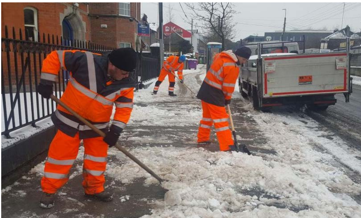
Salting footpaths in Blanchardstown Village Clearing of snow on the Lucan Clonee Road
