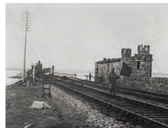
Repairing the viaduct bridge at Malahide after damage caused by the IRA in January 1923
