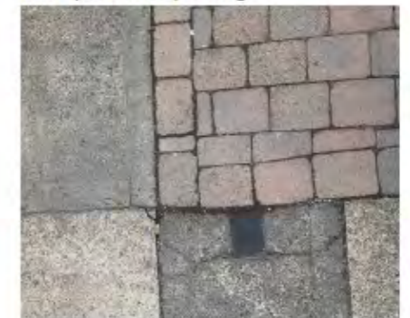
Poor and inconsistent paving materials
