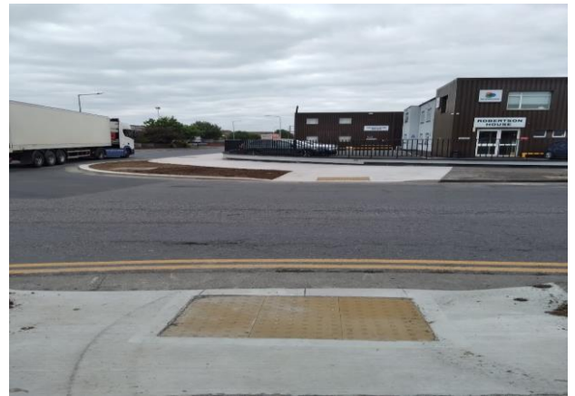
Upgrade works and footpath replacement works, Baldoyle Industrial Estate on behalf of Property Section.
