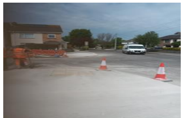
Completion of Kerb Build out and tactile installation in Grange Park Baldoyle
