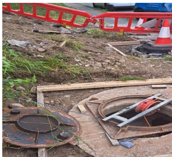
Drainage Rehabilitation works carried out on the R132 between Pinnock Hill and Cloghran Roundabout.
