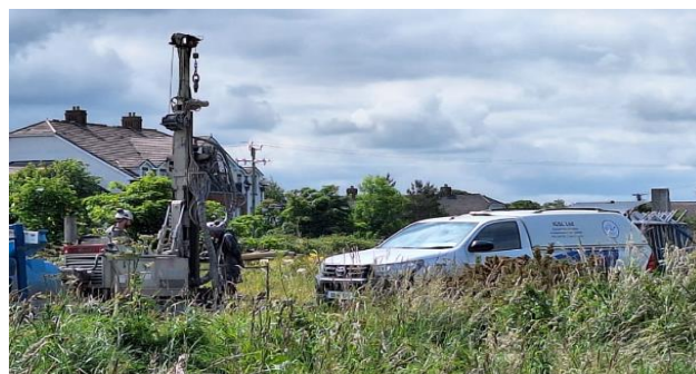
Ongoing Ground Investigations to inform the design of the structures along the route
