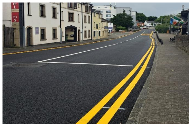
Capital funded road resurfacing works took place on the R125 from Swords Fire Station to the Estuary Roundabout. Below are photos of quality checks being carried out during works.
