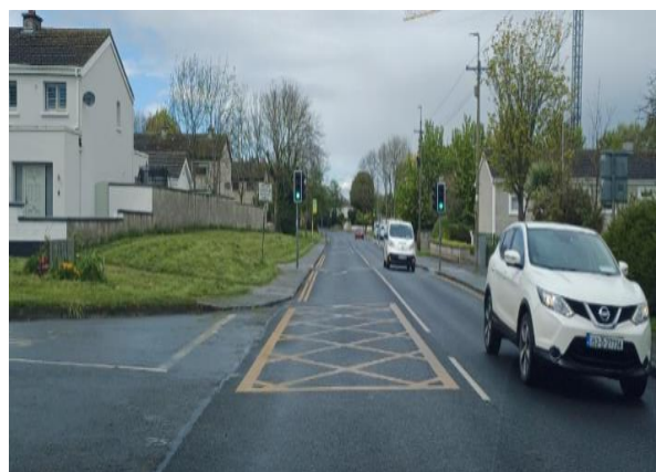
Rathbeale Road – The installation of a yellow box at the junction with Abbeylea
