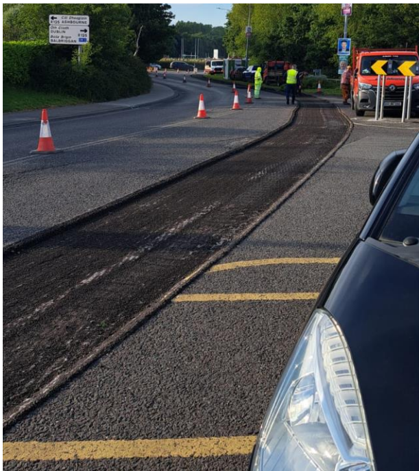
Resurfacing and re-lining Works on North Street, Swords as part of the Capital Works programme 2024
