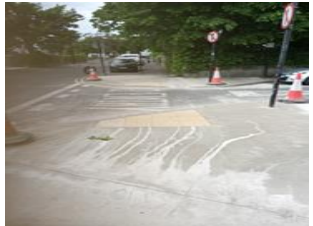
Bath Avenue/Grove Road Malahide: Installation of uncontrolled pedestrian crossing at junction (before, during and after)
