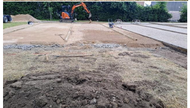
Two new boules pistes have been constructed in Alden Park, Bayside, as part of the 2024 Programme of Works
