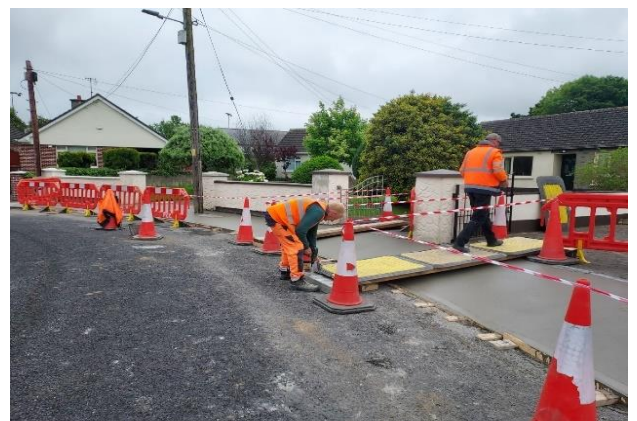
80 metres of footpaths replaced in New Market Green, Balbriggan by the Direct Labour Crew and Fancourt Construction Crew as part of Balbriggan's Footpath General Maintenance renewal programme.
