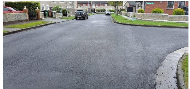
Mooretown and Castlegrange; Road resurfacing works carried out as part of Revenue funded Programme of Works.
