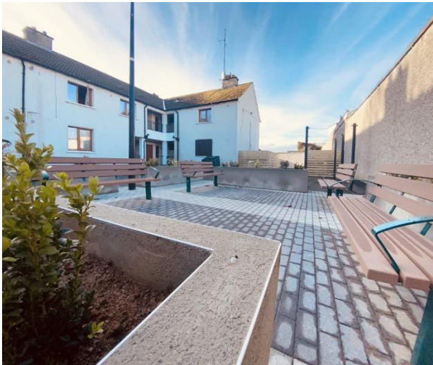
Before and after photos of recent Estate Enhancement Works at Dublin Street Flats
