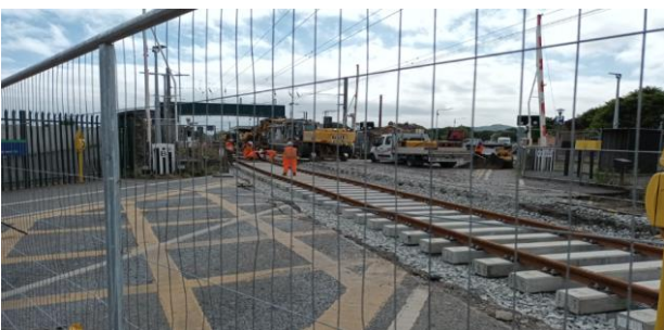
Howth/Malahide section facilitated the full Road closure of Station Road – Sutton for essential maintenance works at DART controlled barrier crossing beginning 22 nd June Saturday Midnight to Monday 24 th June 6AM). Traffic Management issues which occurred during the closure have been brought to the attention of Iarnrod Eireann.
