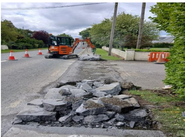
Alterations made to entrance on R127 Skerries Road to address a drainage issue. Works carried out by the Roads Crew.
