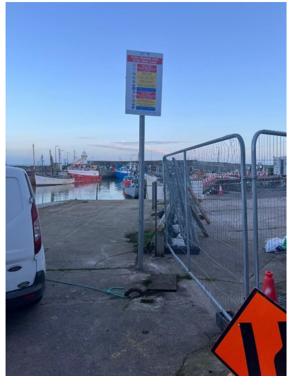
Trip hazards on Balbriggan east pier marked with yellow box around them to highlight their presence.
