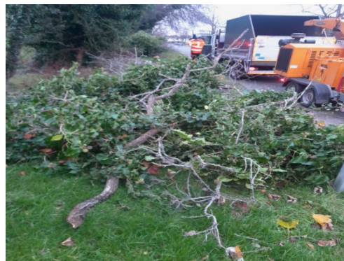
Clonsilla Road, Trees removed
