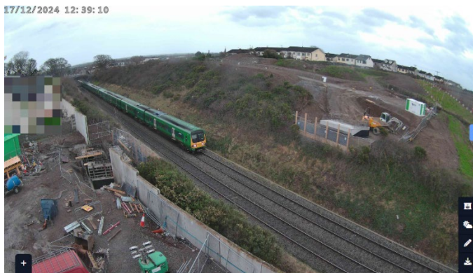
Image of the works site east and west of the railway from the camera installed to capture the works
