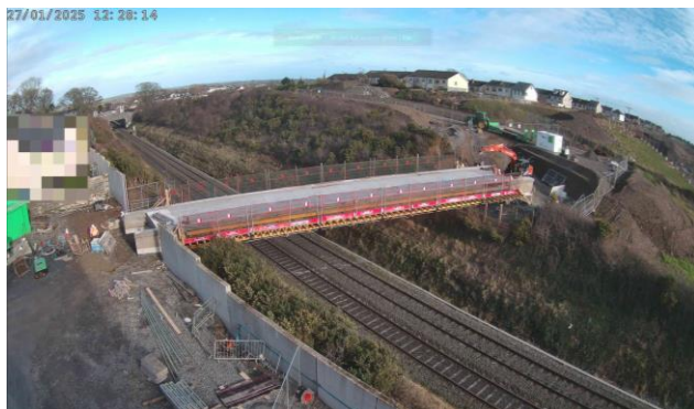
Image of the bridge and works area east & west of the railway from the camera installed to capture the works
