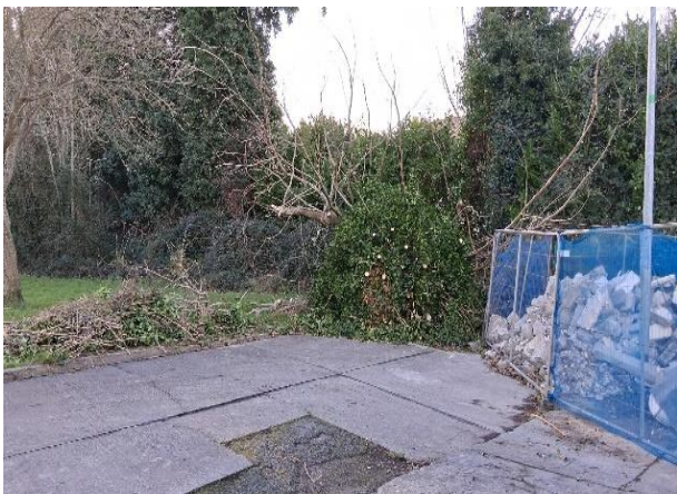
Cut Back to allow access to property and cleaned and processed on Monday.
