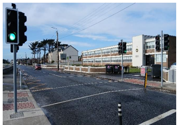
Completion of civil and 95% of Electrical works of Toucan traffic Signals-Dublin Road by St Fintan's Secondary school.
