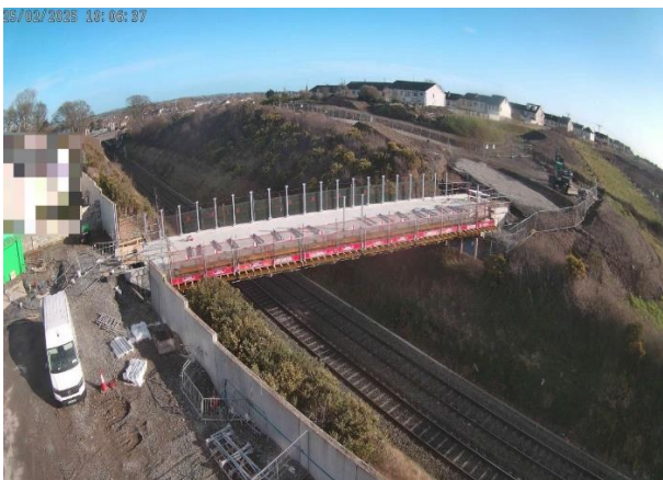
Image of the bridge and works area east & west of the railway from the camera installed to capture the works
