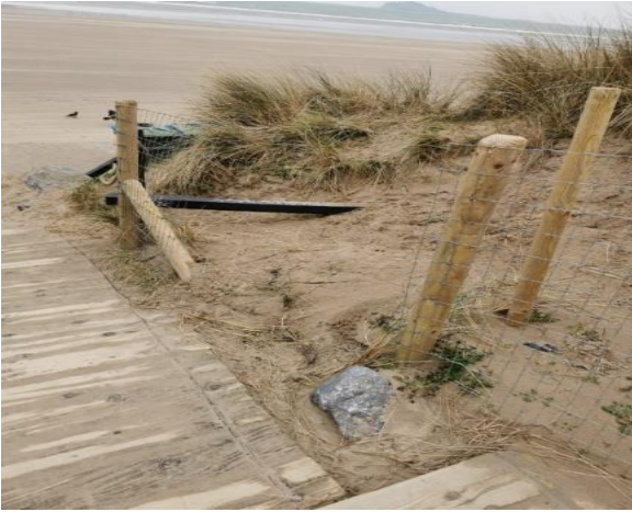
Recent damage to the dune protection fencing Portmarnock Beach.
