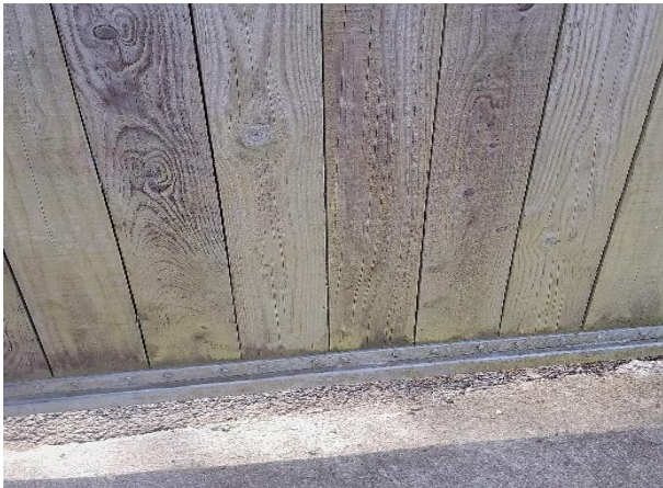
Timber fencing before cleaning.
