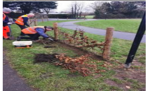
Hedge planting works carried out in St Catherine's Park along fence at carpark
