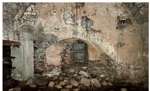
Fig6 Before - vault and lintels requiring repair/replacement
