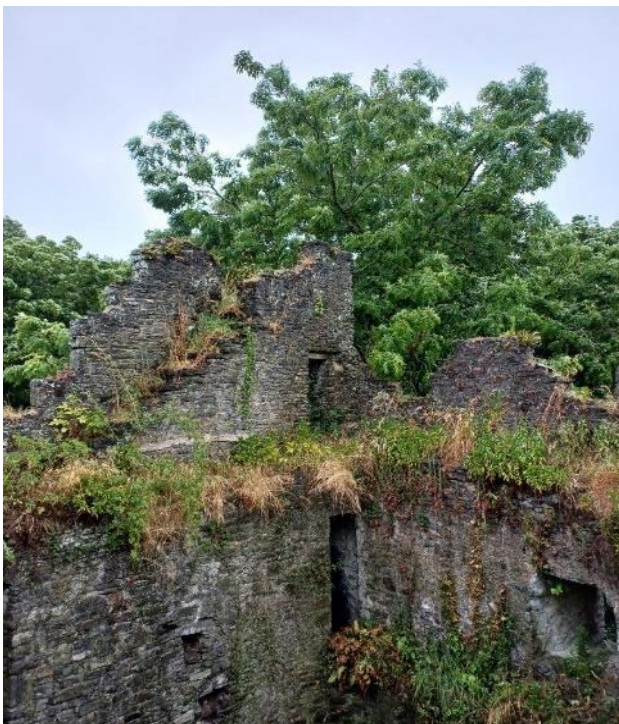
Fig4 Extent of vegetation growth on/in the structure
