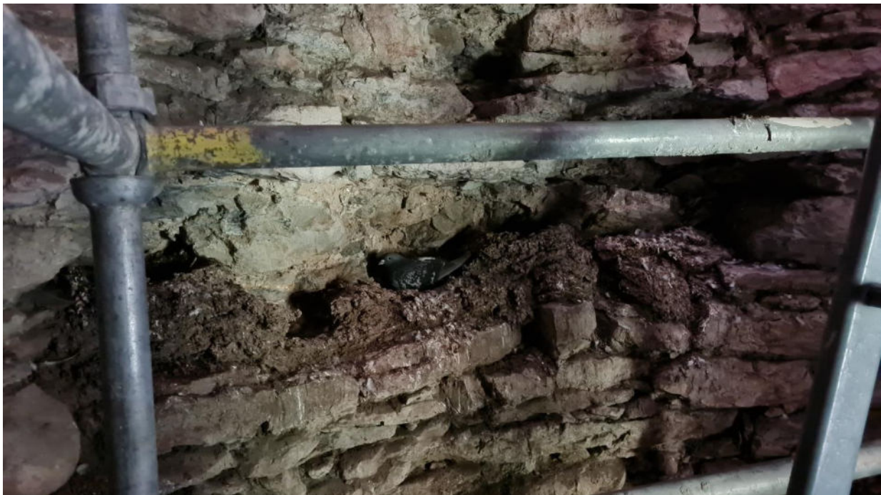
Plate 9: Stone loss resulting in ledges at the same level as the beam holes, note pigeons and nesting material
