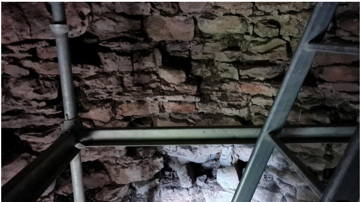
Plate 4: Holes in the wall, west side, above the level of the corbels
