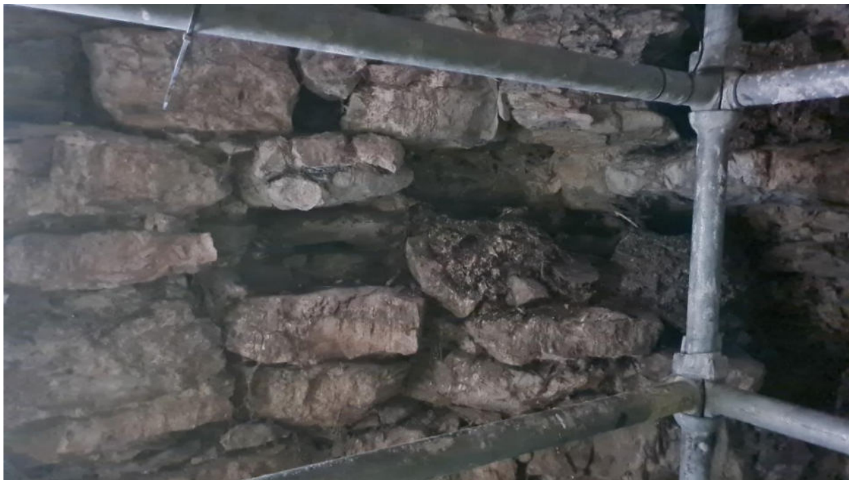
Plate 10: Stone loss on the east side. Possibly caused by the insertion of later wooden beams, now removed.
