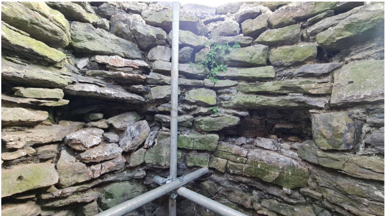
Plate 19: Beam holes 4 (left) and 3 (right), before re-pointing. The distance between these is 1.40m.
