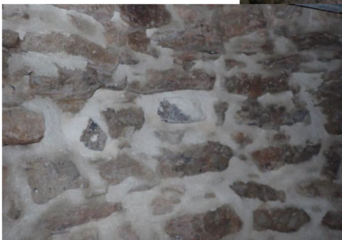
Plate 7: Beam hole 3 before and after re-pointing; stones were in the hole, and they were mortared in position in error.
