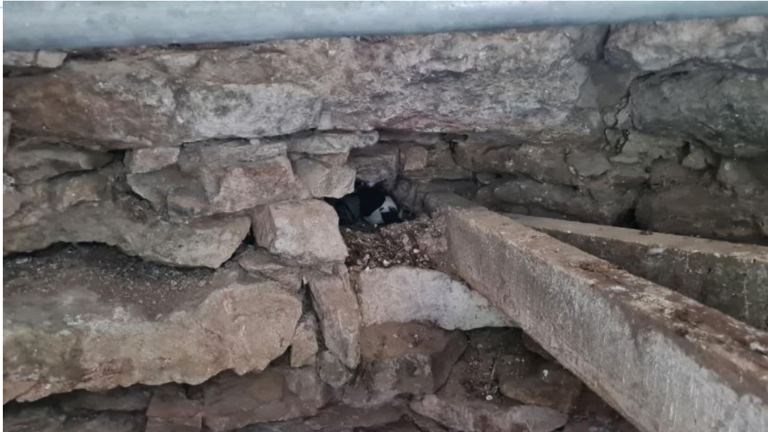
Plate 12: Beam hole 4 with pigeons in situ on build-up of soil and droppings, and two wooden beams inserted into it
